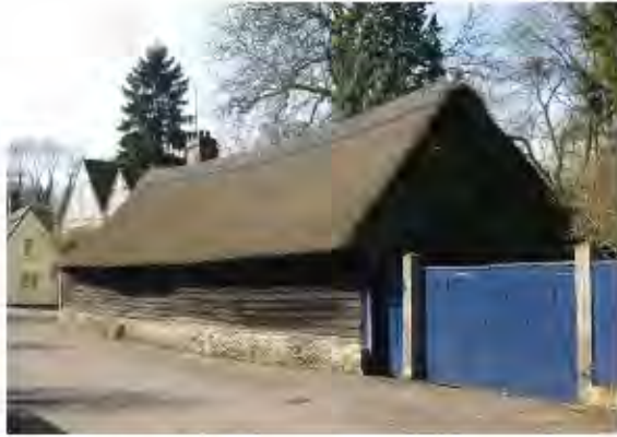
Image 12a. Natural timber black tar weatherboarded barn Typical in Linton's CA and the locality
